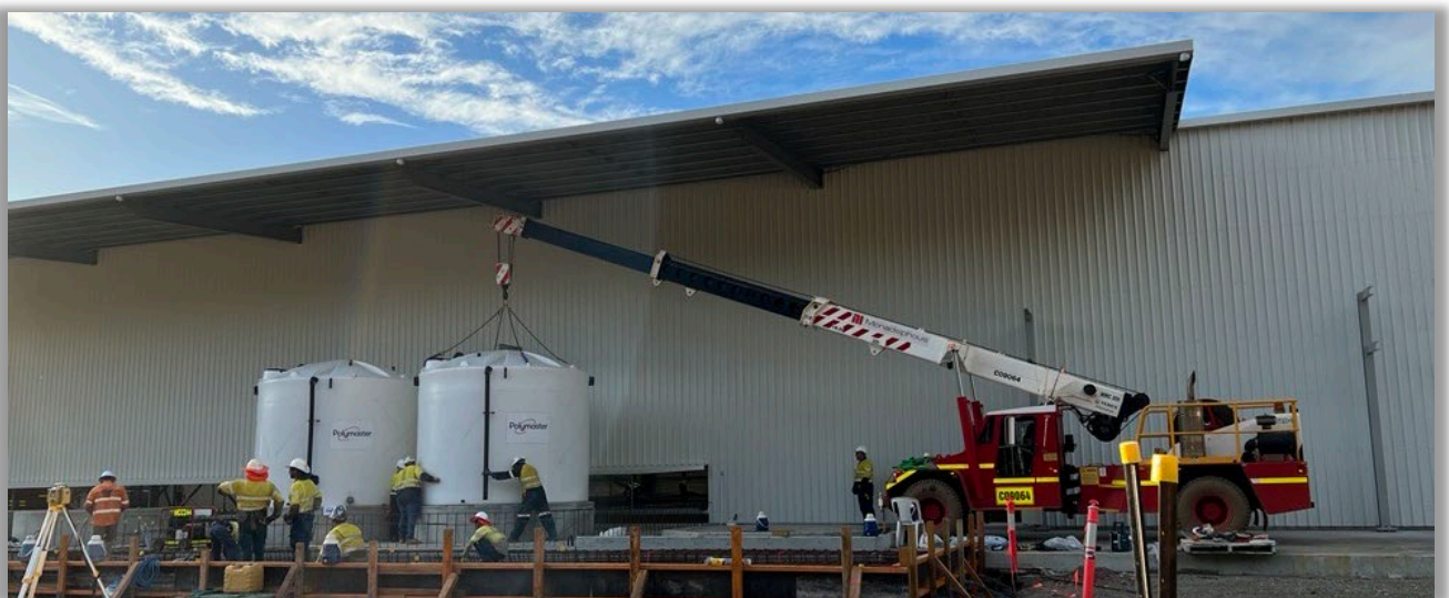
Installation of PPF reagent tanks
